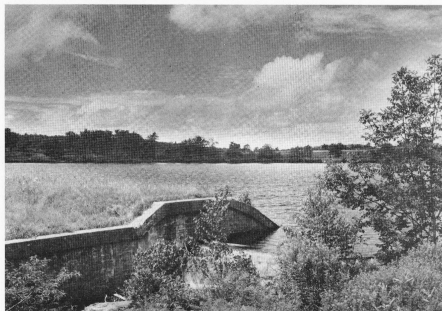
The above picture was taken recently of the Chestnut Hill Reservoir showing the rain-swelled water running over the flashboard which is twelve inches above the spillway. Comparing the level of the water now to last year about this time we find that it was nine inches below the spillway. The reason is of course that we've had a lot more rain this summer than last.
